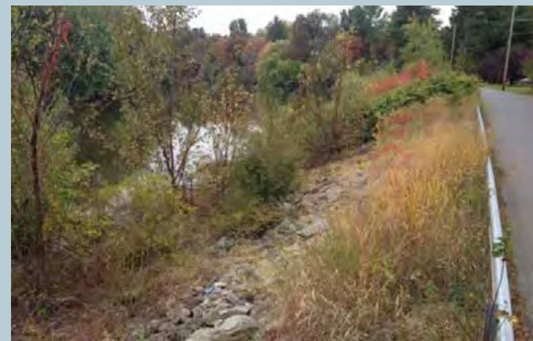
Living shoreline constructed by ACOE on the Wallkill River in Rosendale, NY - mix of boulders and vegetation.
