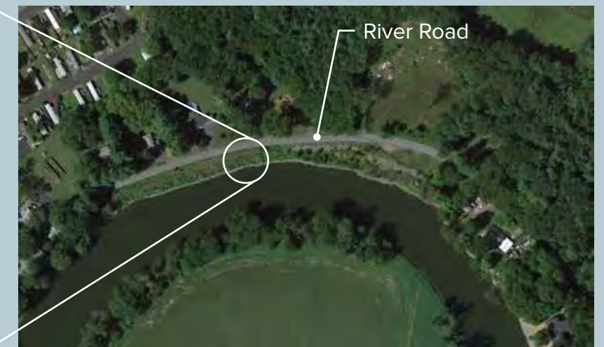
Living shoreline on the Wallkill River in Rosendale, NY. By 2004, the river had reached and was undermining River Road.
